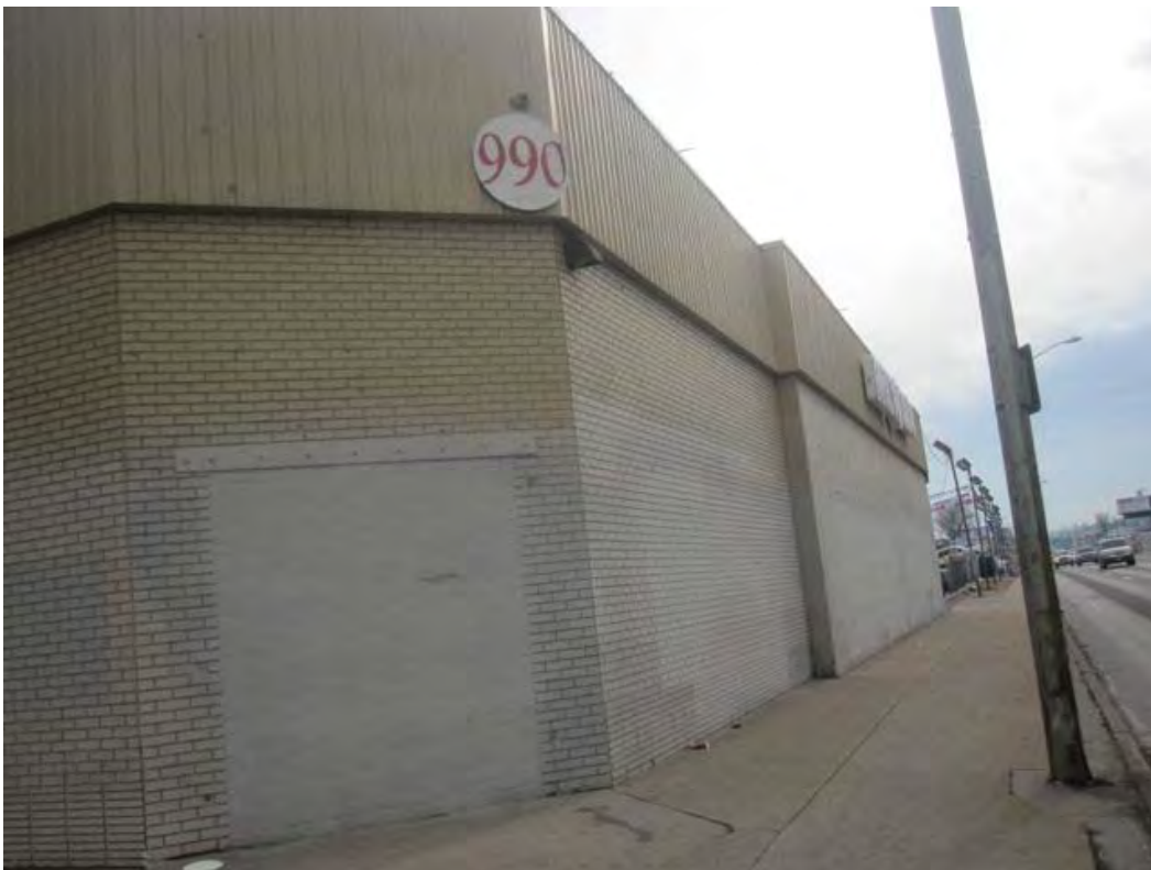
Photo 5DV11365_4 Looking southeast at west elevation and former corner entrance that has since been enclosed.
